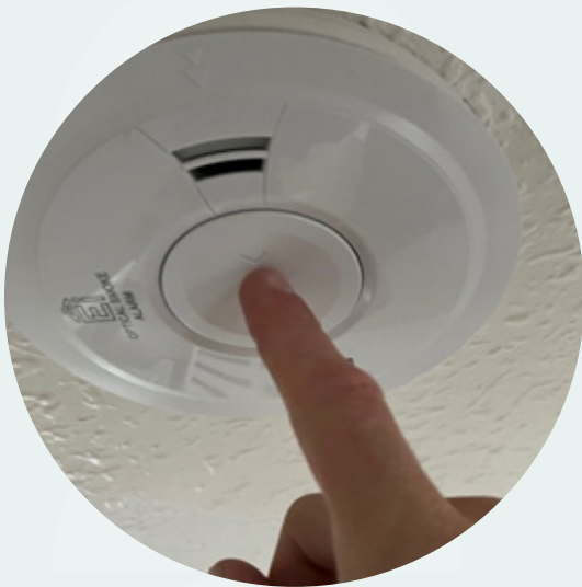
Testing a smoke alarm
