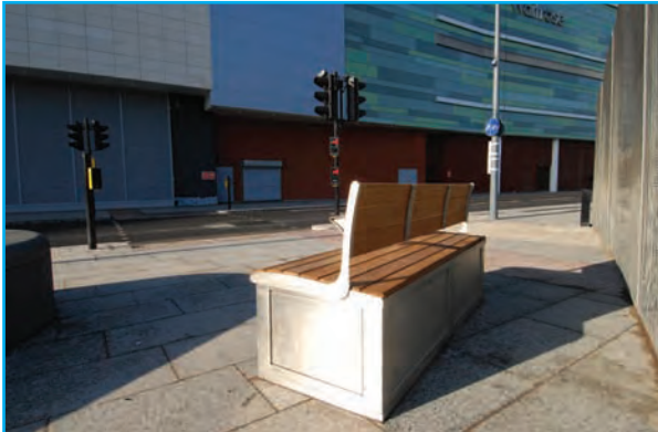
Bench containing traffic signal controller
